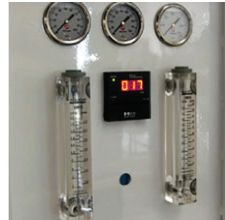
The controller installed in a commercial system
